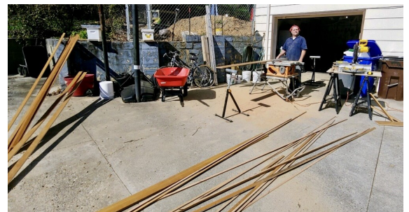
Wood from old pews is being used for molding for the new offices.
